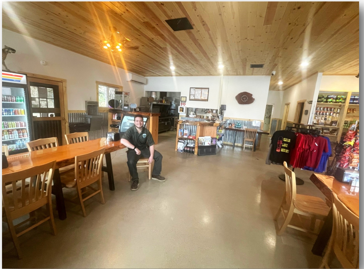
Clear Lake Ranger Devin Kress shows off the newly remodeled lodge/restaurant featuring live edge tables, corrugated metal wall coverings, knotty pine ceiling and trim and epoxy flooring and new counters.
