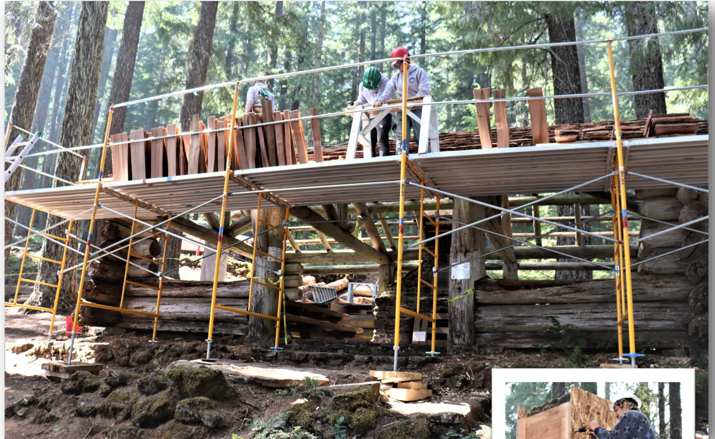
HistoriCorps volunteers install new hand-split cedar shakes on the picnic shelter at Clear Lake Resort.
