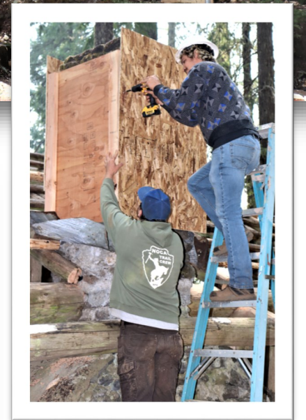
HistoriCorps staffers Jason Benson, left, and Remy Buxton, work on the picnic shelter’s rock chimney.
