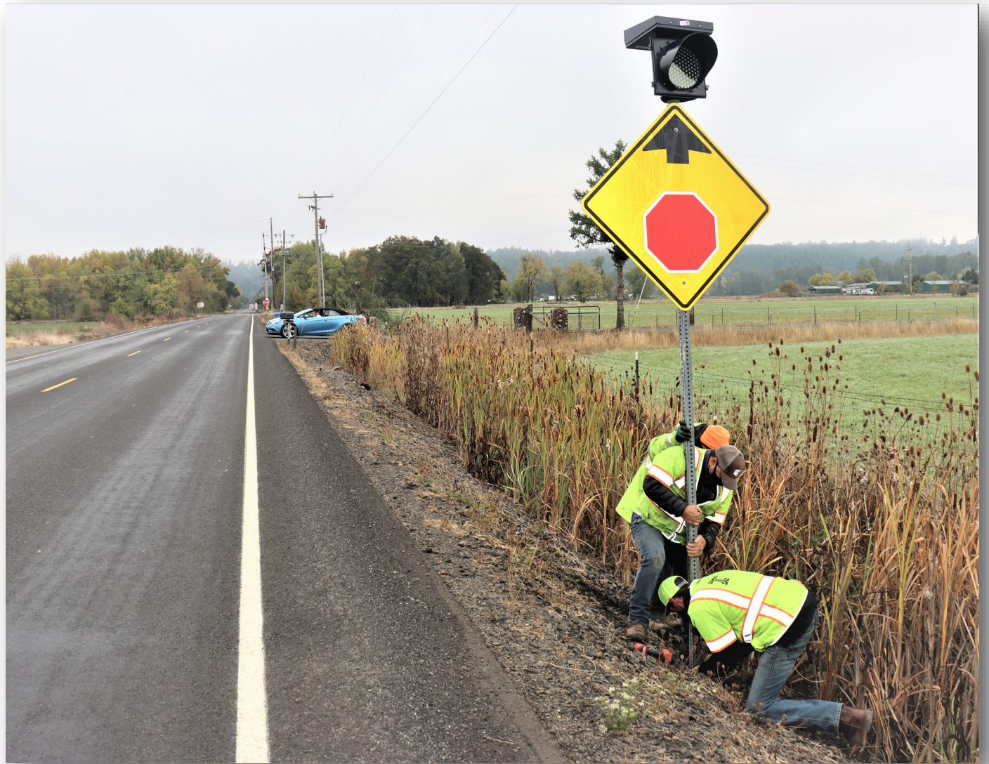
Billy Kelso, center, Robert Giles and Jarrett Clark of the Oregon Department of Transportation prepare and install a new solar-powered advanced warning flasher on Richardson Gap Road south of the Highway 226 intersection. The driver of the vehicle in the background rolled down her car's window and thanked them for their work.
