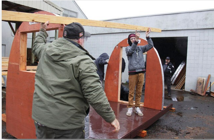
Kobe Pangle, right, and Sweet Home High School instructor Will Coltrin inspect the fit of a rafter on a newly erected Quonset-style hut to be placed at a homeless shelter site east of Bi-Mart. Coltrin's advanced construction class worked to assemble the structures.
