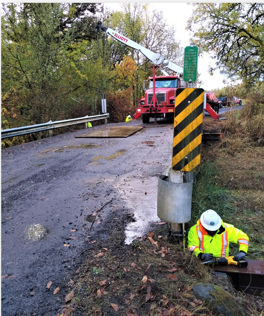
A Linn County Road Department bridge crew worker replaces a cap on a bridge on Glass Driver, south of Tangent.
