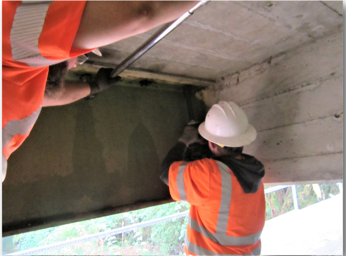
Above: Road Department staff install shear studs on a bridge on Lulay Road near Scio.
